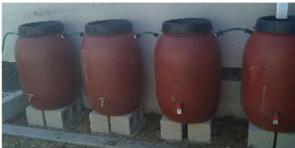
Figure 12. Example of rain barrels connected in series to a single downspout.
