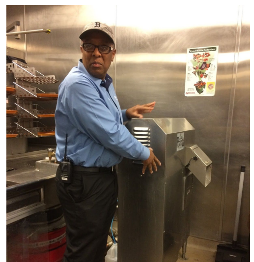
Charles pointing out the pulper, a machine that chews up food waste so that it can be sent to an industrial composting facility.
