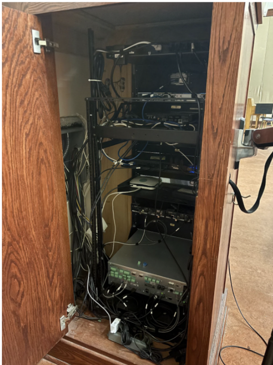
Photo 3: Old technology box in Kaplan A48
